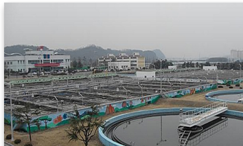
Gyeongju sewage treatment facility
